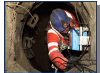
Waste Water Monitoring
